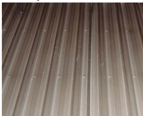
Garage Wall - Exhaust Soot - Before
