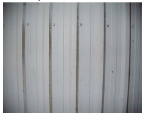
Garage Wall - Exhaust Soot - After
